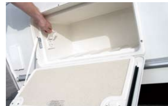
Mains socket in wet locker
